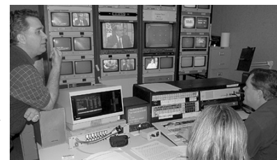
Bob Heyl (left) joins Kathryn Griffith in the control room.
